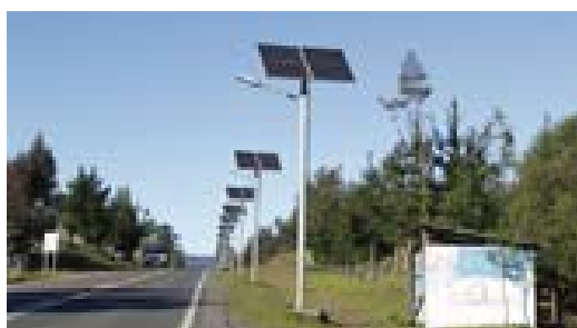
Intelligent solar single lamp project in Delingha Economy Industrial Park, Qinghai
